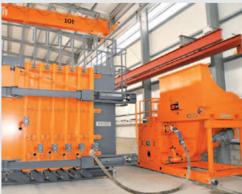
Hydraulic battery system with pump car
